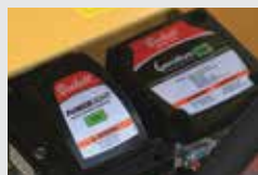
Diesel fired Beckett Burner
